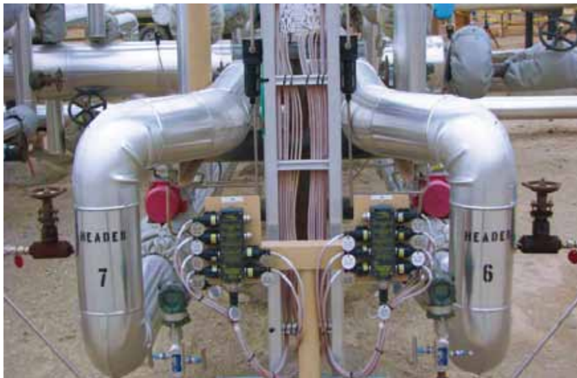
Foundation Fieldbus field elements
