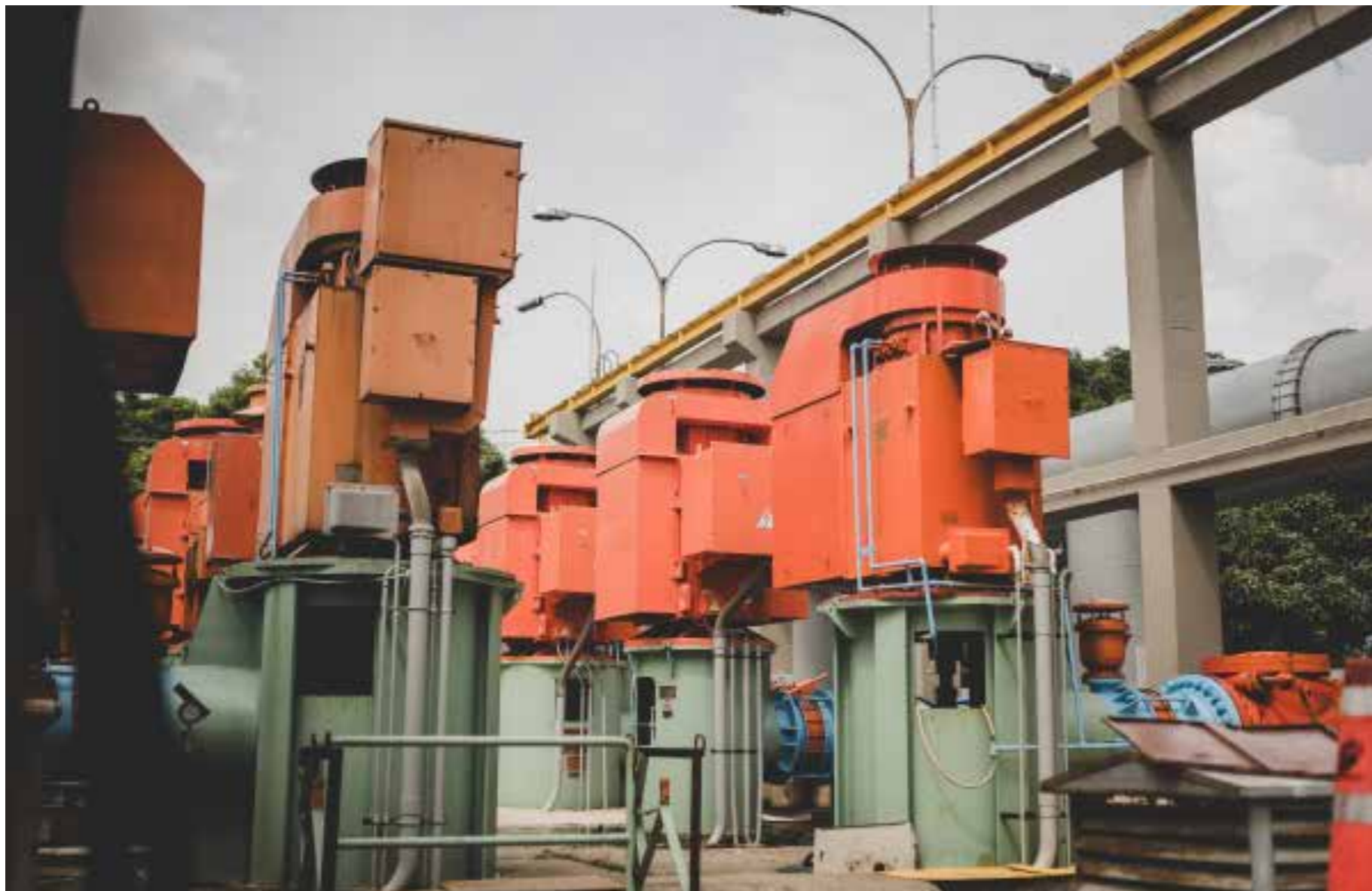
Optimization of drinking water treatment plants in Cali Colombia
