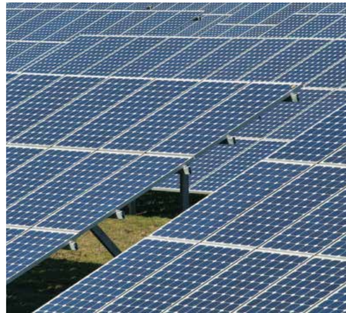
Intipampa Photovoltaic, Peru
