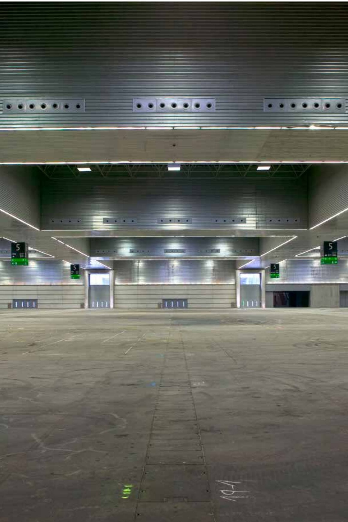
Bilbao Exhibition Centre. The great volume and its diverse, complex usage, condition the design of MEP building services which are solved by giving flexibility and reliability to the systems.
