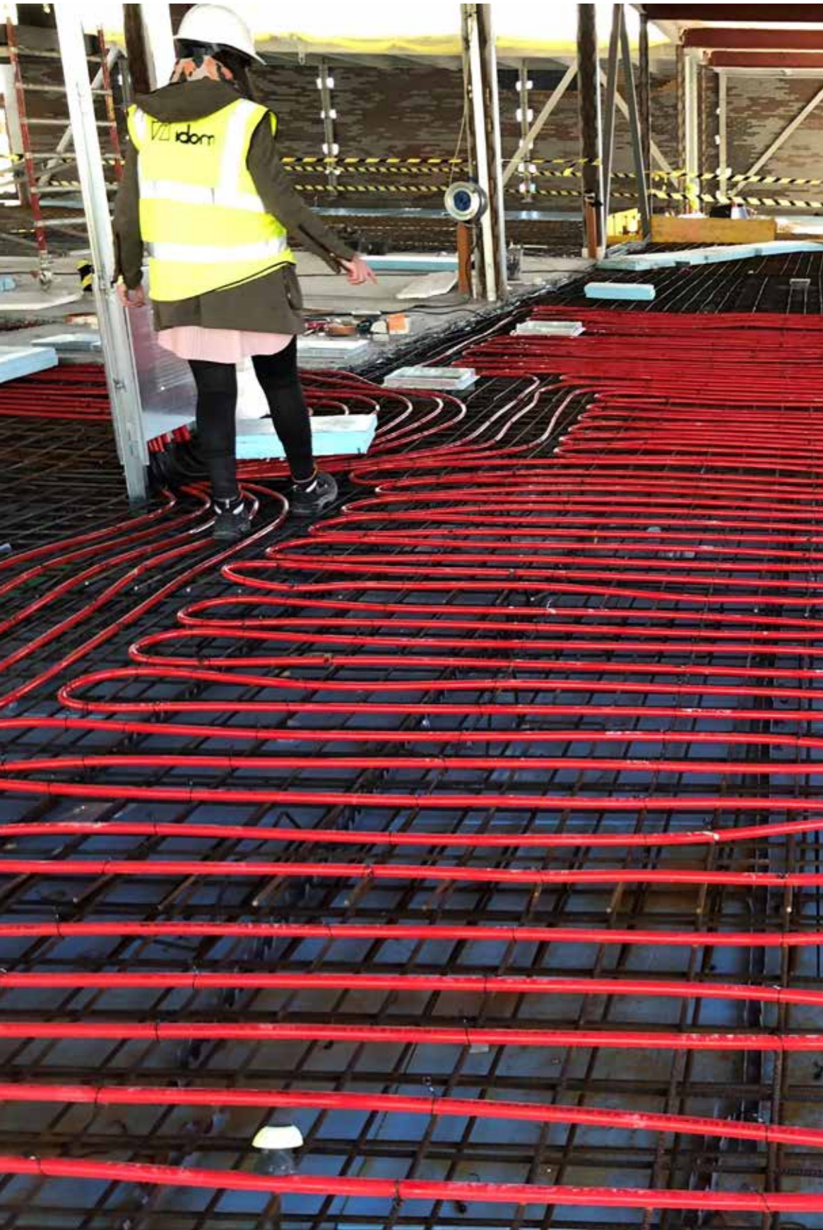
Energy thermo-activation in a building of the New Red Elctrica Campus in Tres Cantos (Madrid)
